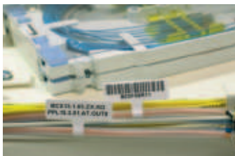
Fibre optic cable markers
