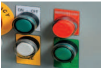
Control panel labels
